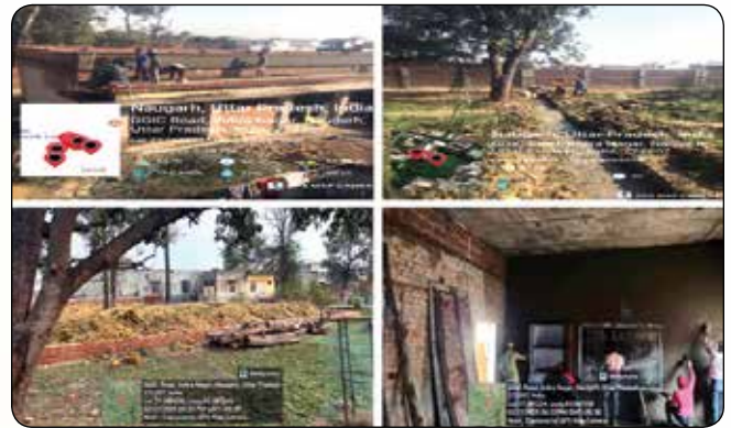
CSR support for Government Girls Inter College(G.G.I.C), Siddharthnagar, Uttar Pradesh towards strengthening the infrastructure of college building
