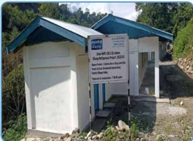
Construction of Boys and Girls Hostel for Govt. Residential School Ranli, Dibang Valley, Dibang Multipurpose Project, Arunachal Pradesh
