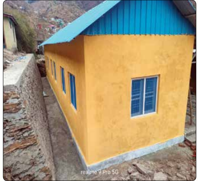
Construction of 03 no. additional class rooms in Govt. High School Barmota, Bani (Resolution of Gram Sabha Panchayat Barmota), Kathua
