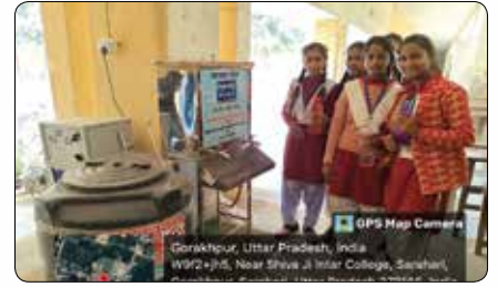
Installation of 15 Nos Reverse Osmosis (RO) Water Treatment Plant 'Swachh Jal Dhara' at schools in District Gorakhpur of Uttar Pradesh
