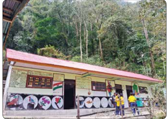
Renovation, beautification and misc. works at Government Senior Secondary School, Pheedang, South Sikkim
