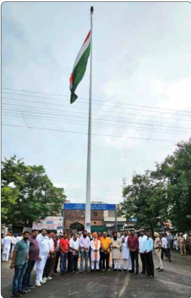
Installation of 100 Feet National Flag with Decorative Foundation at Railway Station Sunam, Village -Sunam Udham Singh Wala, District – Sangrur, Punjab
