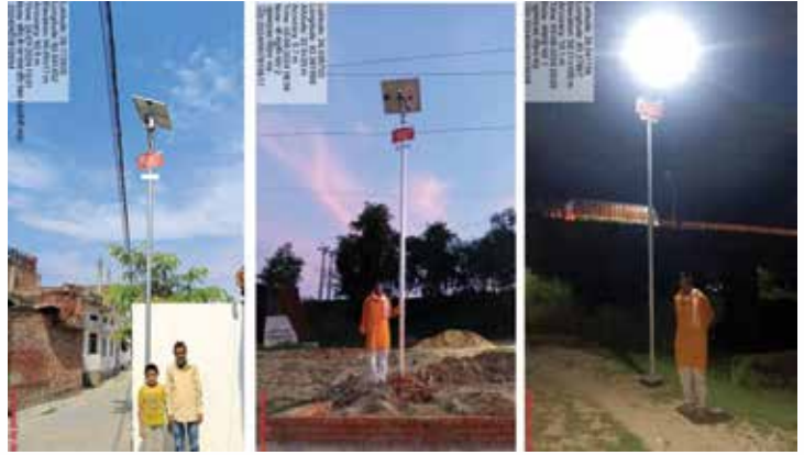
Installation of Solar Street Lights in Village Kazha, Tehsil-Mohammedabad, Block - Raniganj, District-Mau, Uttar Pradesh
