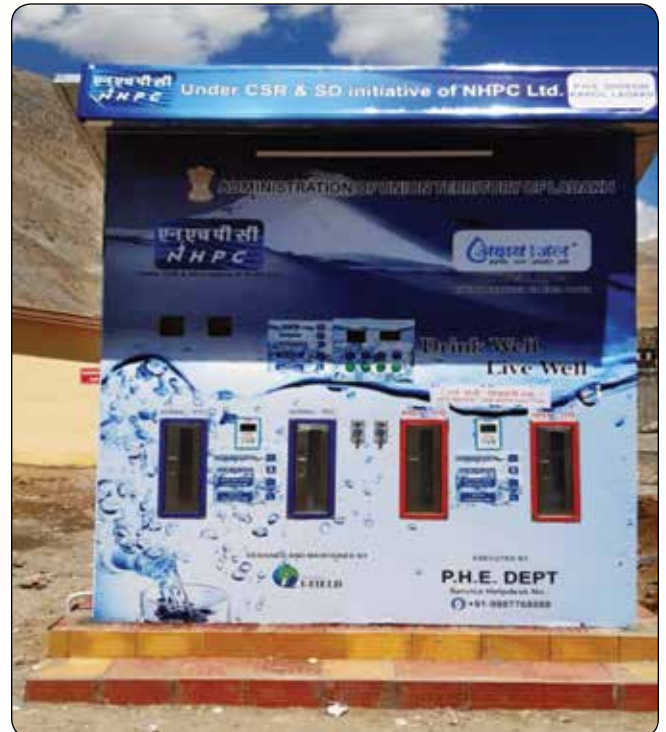
Installation of water ATM of 250 LPH at New District Hospital, Kurbathang, Kargil
