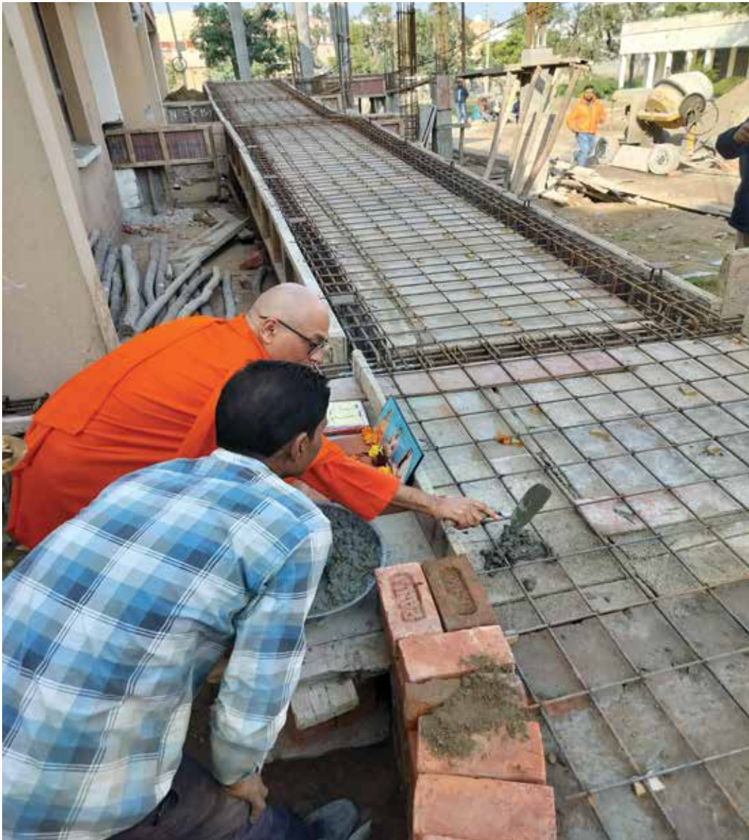
Setting up an eye care unit, repairing and remodelling of the Eye OT, Construction of Ramp with Canopy at Ramakrishna Mission Medical Centre, Jammu
