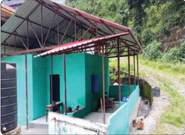
Construction of Mid-Day meal Kitchen and electrification in the Govt. Sr. Sec School, Dickchu, Gangtok, Sikkim
