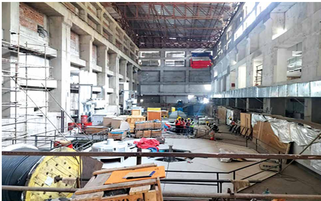
POWER HOUSE – 120 MW RANGIT-IV PROJECT(SIKKIM)
