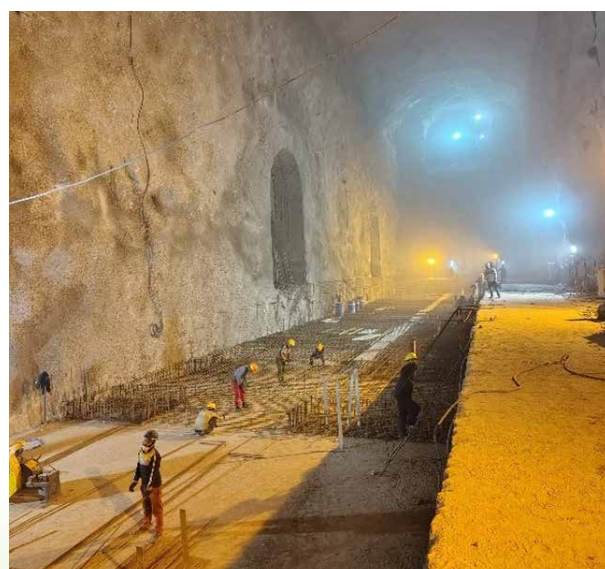
TRANSFORMER CAVERN – 850 MW RATLE PROJECT (UT OF J&K)
