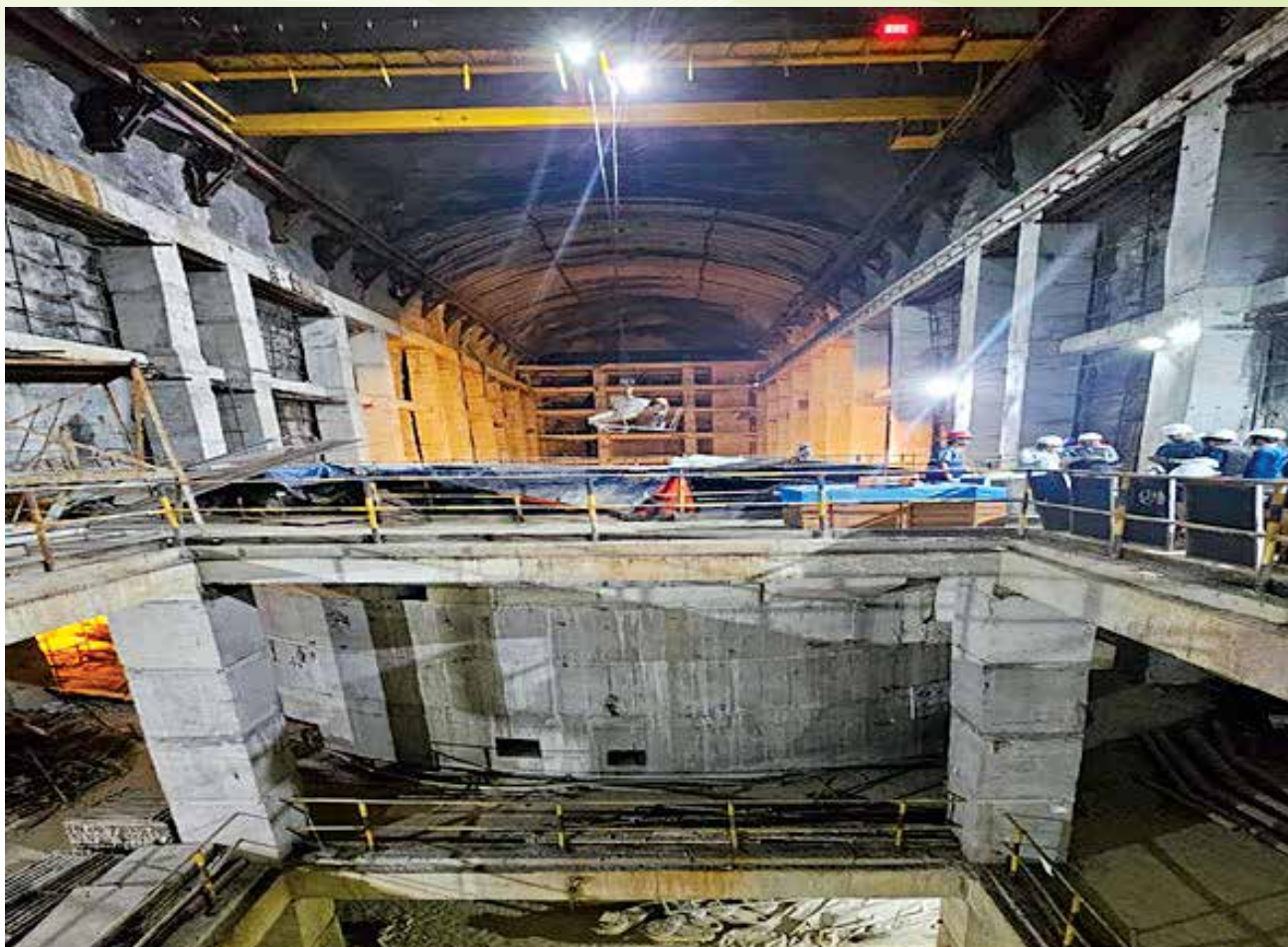
POWER HOUSE – 500 MW TEESTA-VI PROJECT (SIKKIM)
