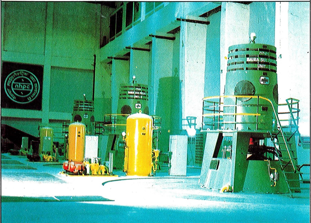
Inside view of power house - Baira Siul Project
