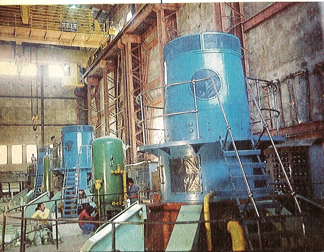
An interior view of power house-Loktak
