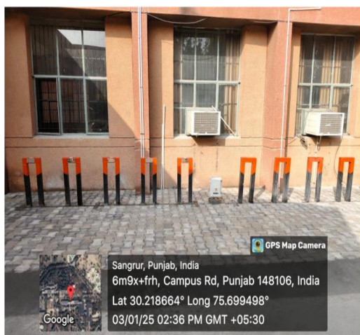
1. (i) Docking Station installed in front of the Science Block
