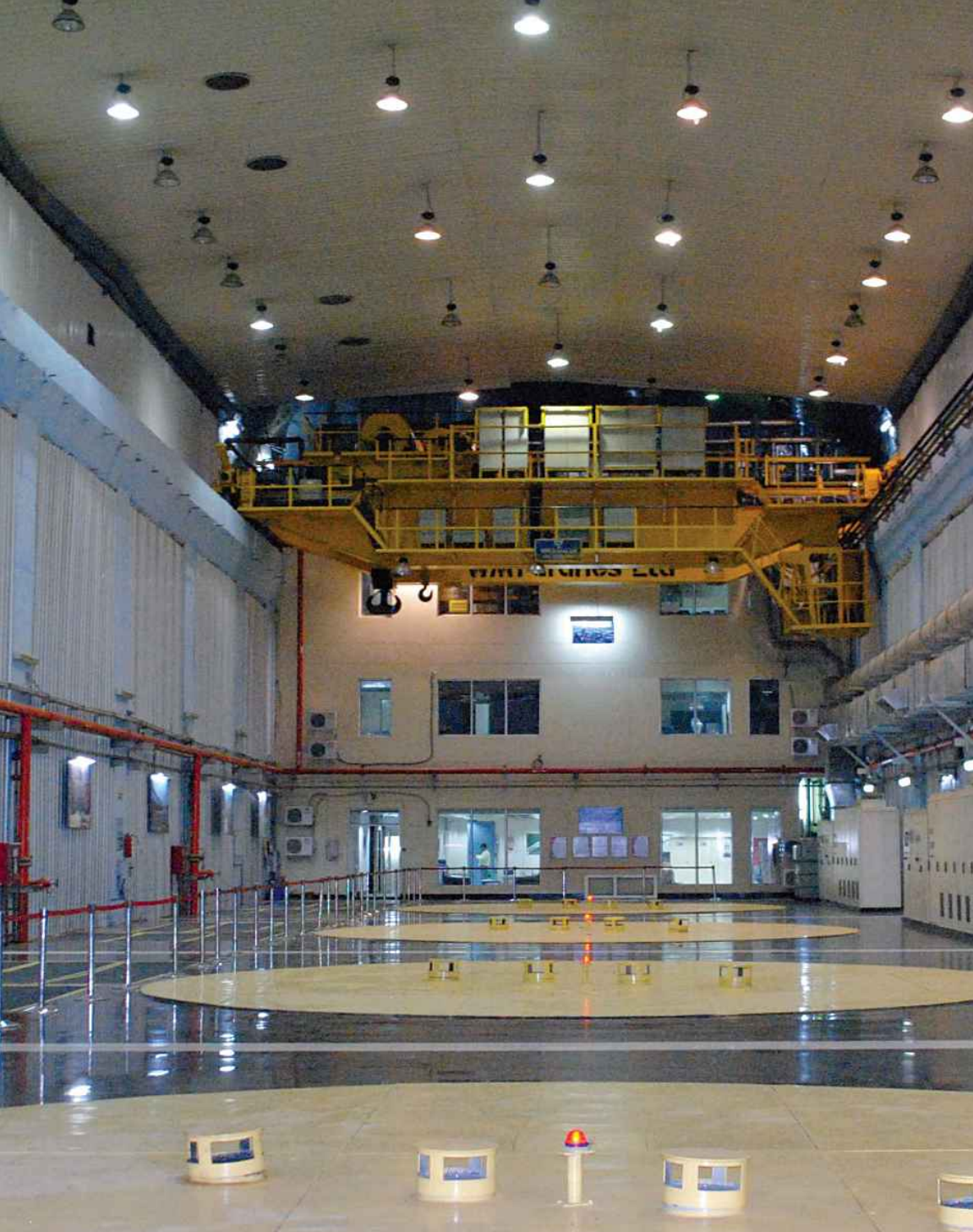
Power House of Dhauliganga Power Station (280 MW), Uttarakhand
