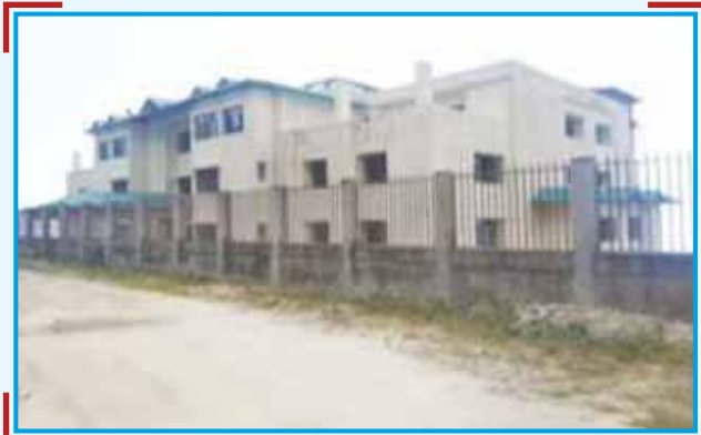
Ongoing construction of the Engineering College at Takdah under support of TLD-III & IV PS)
